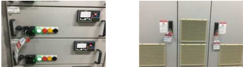
Gambar 4.6 Control Panel & Sub Station
